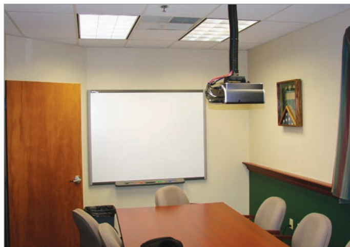
Traffic Planning and Design’s conference room, with ceiling-mounted Canon REALiS SX6 Multimedia LCOS Projector
