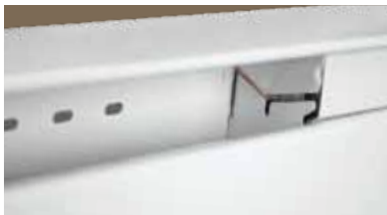
THERMAL PROTECTION HIDDEN INSIDE THE JUNCTION BOX
