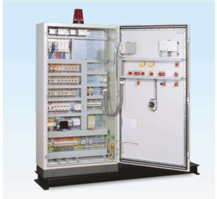
TC 4 installed separately from the system in a control cabinet
