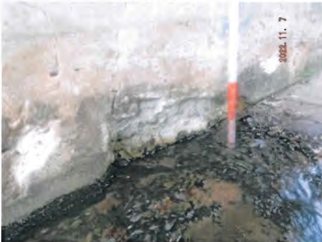
North Abutment Spall (3-feet long by 1-high)
