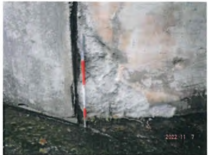
North Abutment, West End Spall (4-ft High by 4- Long and 4-inches deep)
