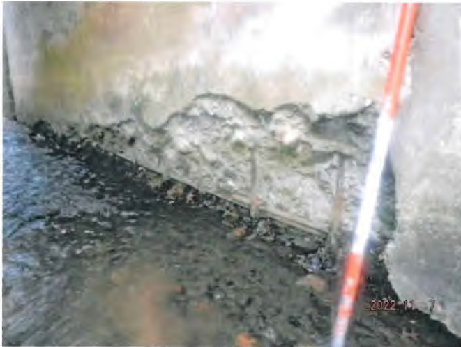
South Abutment Spall (15-Long by 2- High and 5- inches deep)
