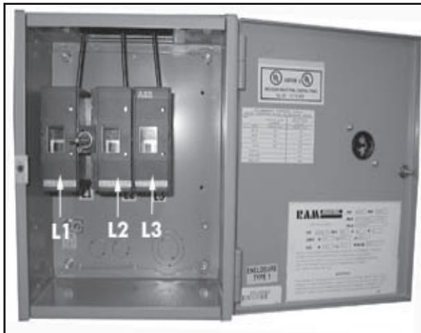
Incoming Power Drive w/Fused Disconnect
