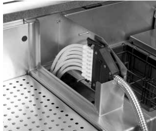
SHA-6 with access cover removed
