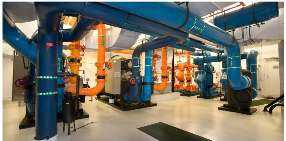
Mechanical equipment rooms are subject to refrigerant leaks ©MSA Safety
