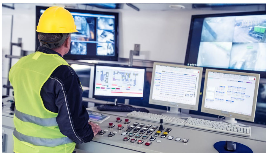
BACnet revolutionized interoperability of building automation devices and systems. ©MSA Safety
