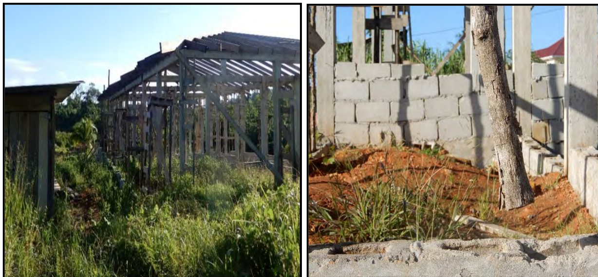
Photographs of the incomplete works and abandoned site
