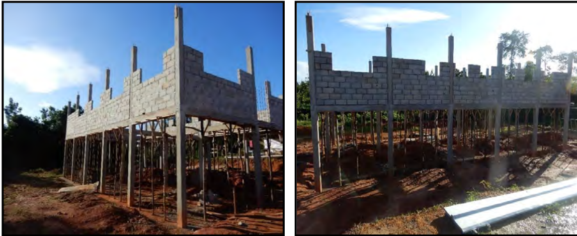
Photographs of the incomplete Education Office
