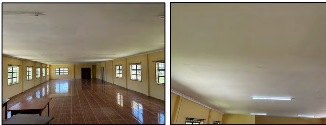
Ceiling works showing moisture damages
