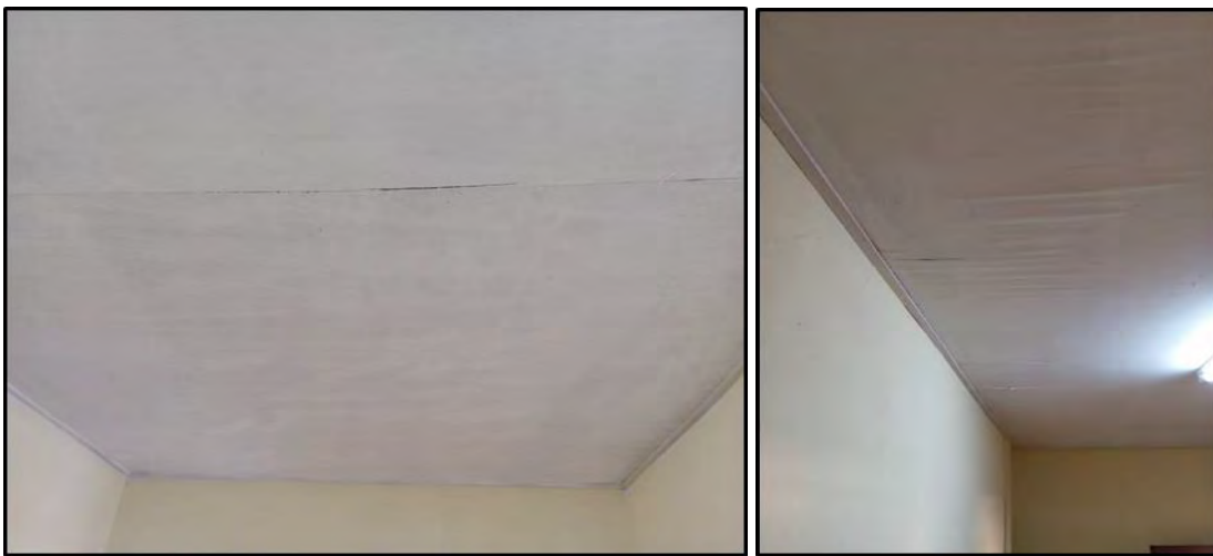
Ceiling works showing moisture damages
