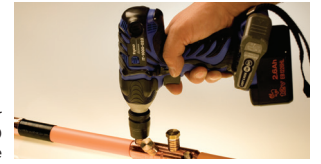
Copper Shearbolt connector installed on EPR insulated 4/0 kcmil 15 kV cable
