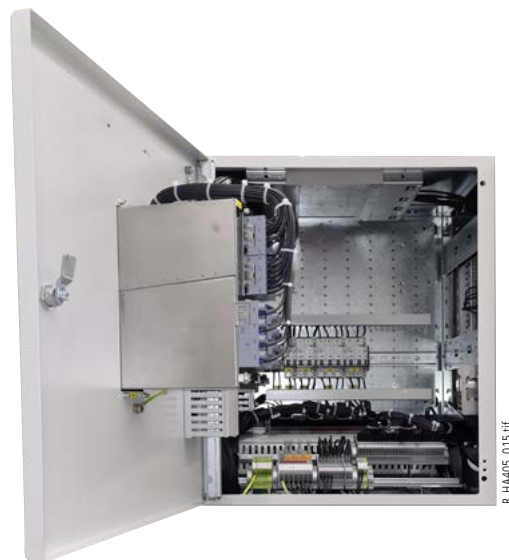
Open low-voltage compartment with built-in equipment (option)
