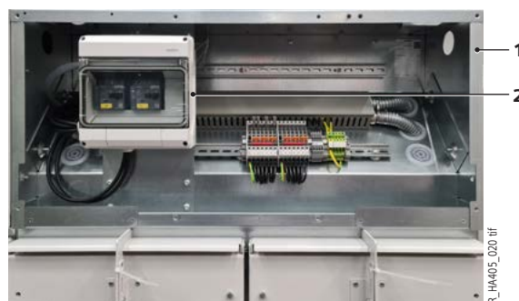
Low-voltage niche of a billing metering panel type M, open cover
