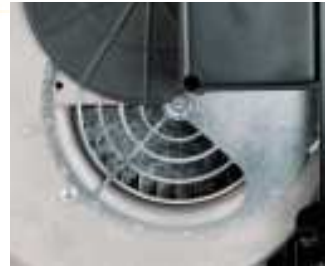
Air damper completely open
