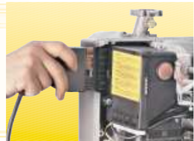
7-pole socket incorporated in the control box
