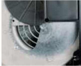
Air damper partially open
