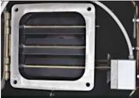
Example of the servomotor and dampers for air setting
