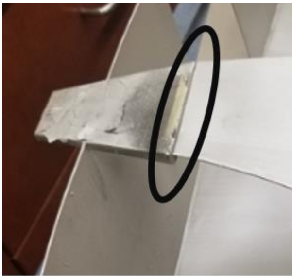
Figure 8.2.1 Repaired Koshelev transformer connection.
