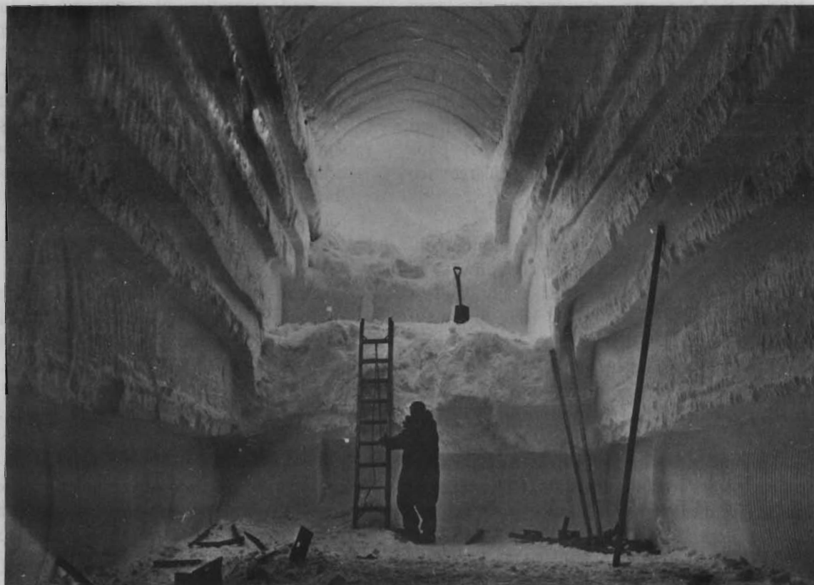
Figure 8-49. Completed Trench With Roof Forms Removed and Ready for Installation of Buildings at Camp Century, Greenland (End-wall treatment to provide for escape hatch is shown in this photograph.) (Photograph by Waterhouse)
