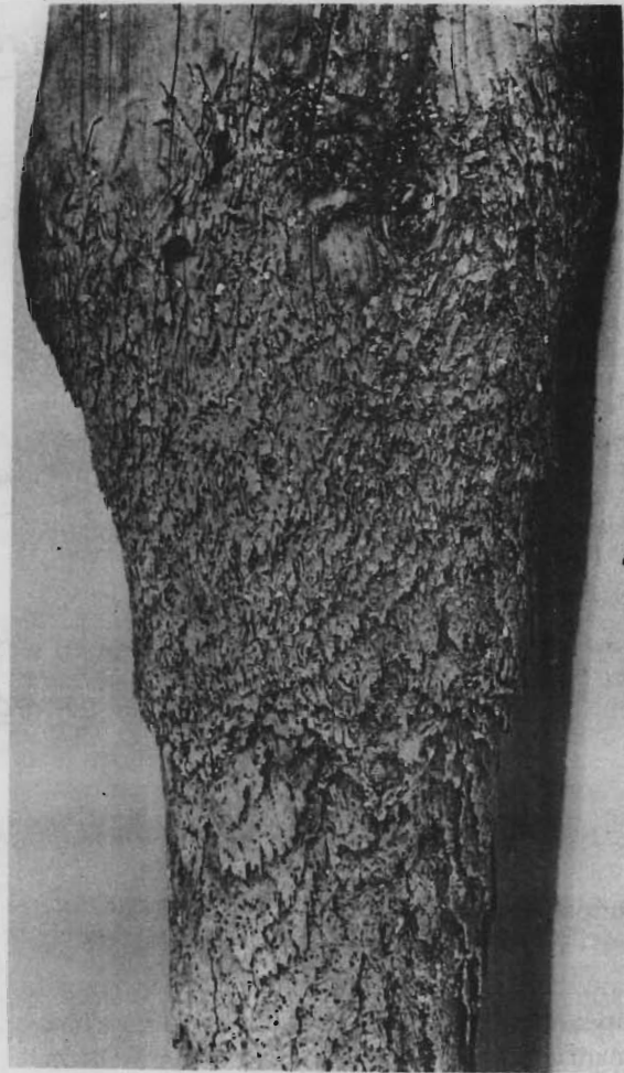
Figure 13-15. Piling Damage by Crustacean Borers ( Limnoria ) (Ref. 6)
