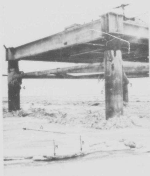
Detailed Ice Failure I, Note the Bern of Broken Ice on Each Side of Path.
