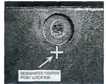
Fig. 4 — A mislocated weld.
