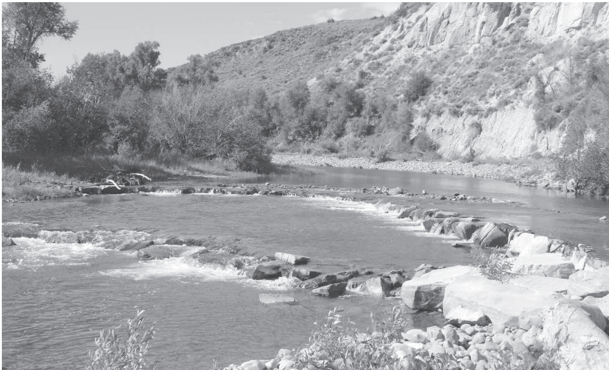
The completed realignment of the Bear River is pictured following removal of the Evanston dam and the addition of rocks to redirect the river and creating a channel for the irrigation canal. (UINTA COUNTY HERALD/Kayne Pyatt)
