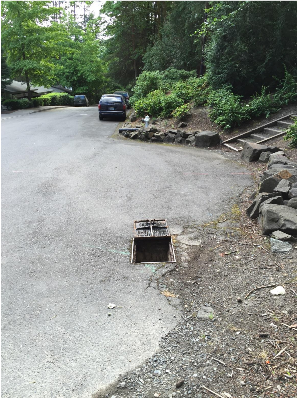
Type 1 catch basin which is the collection point of NDA 3. This catch basin is located within Mine Hill Apartments parking lot.
