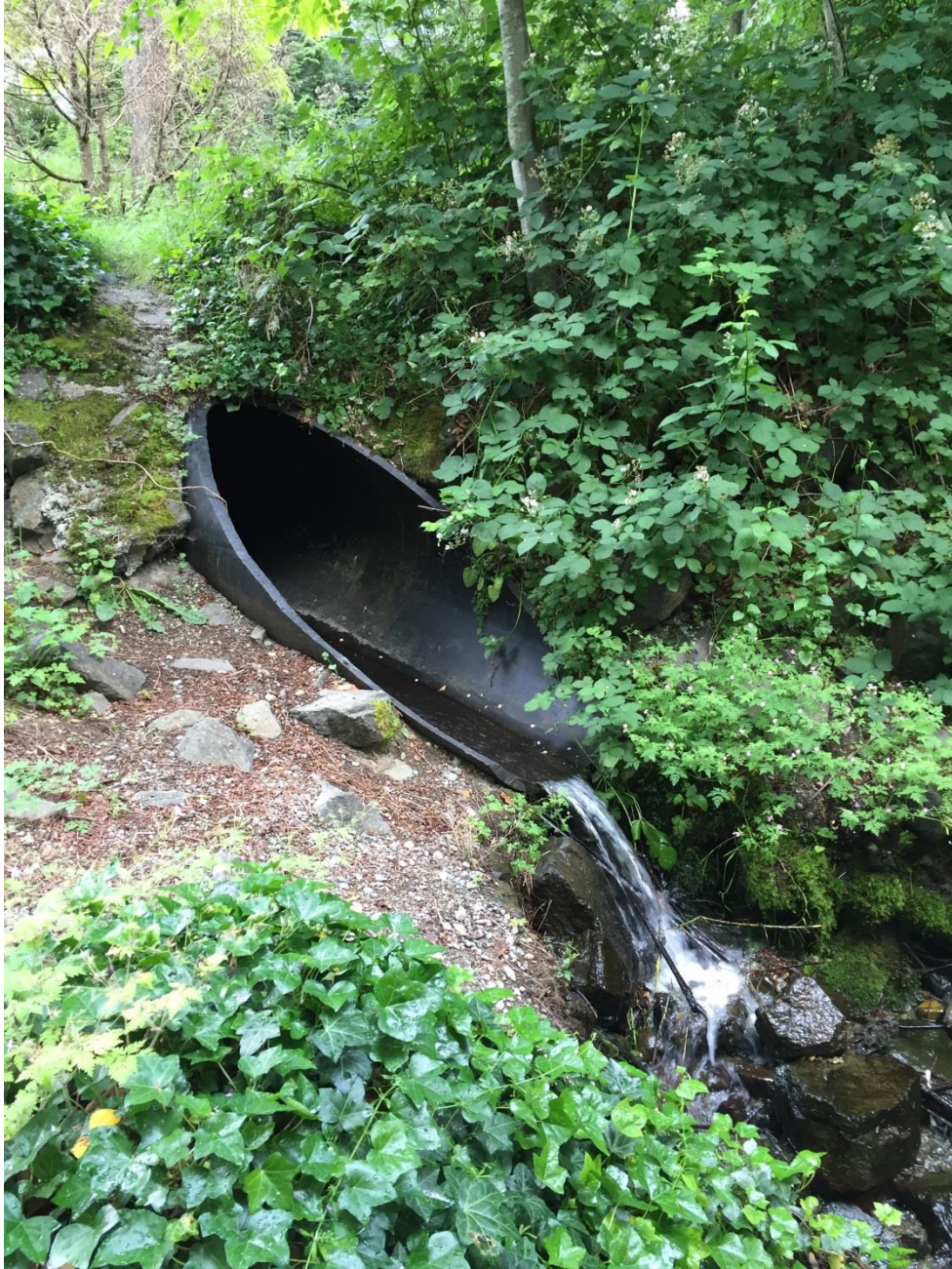
42" discharge point into Issaquah Creek.
