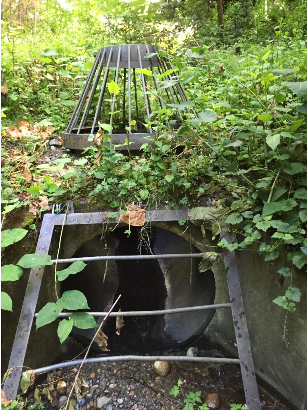
Looking northeast at the northeast 42" diameter culvert conveying Mine Hill Creek in a northeasterly direction.
