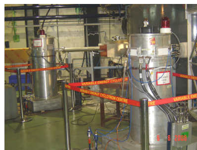
Fig.1. High power rf amplifiers installed at SCC Vault
