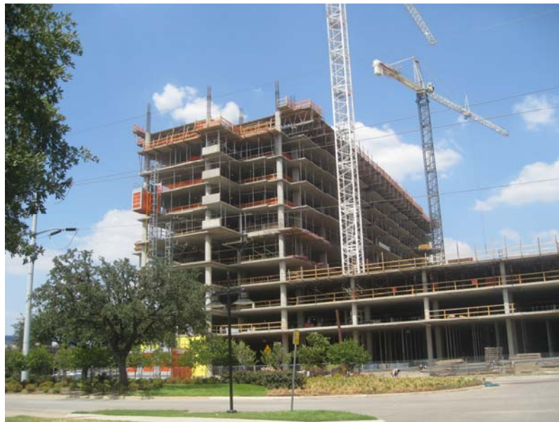
PM Realty’s 1400 Hi Line Drive project under construction. The project includes extending streetscape improvements along Edison Street and the Hi Line Drive/Stemmons Freeway underpass connecting to the Victory area.
