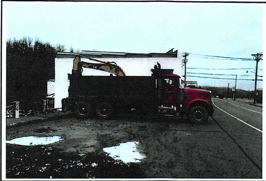
1/5/2017 – Rt. 19 North Weston Old Giovanni Restaurant and Laundromat location; Mainline LLC on location.
