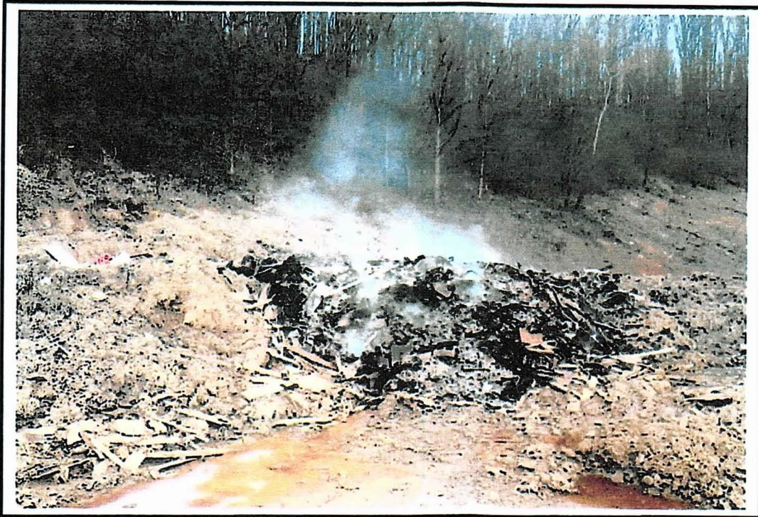
1/5/2017 – Construction/Demolition waste burning at the old Savin Lumber property owned by Mr. Kevin Lee.
