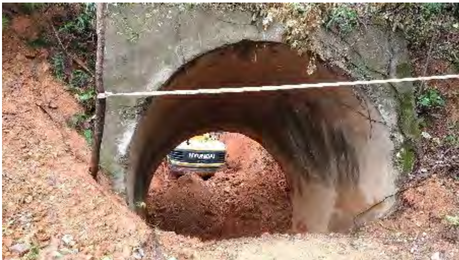
Figure 10.1: The Remains of the Concrete Collar of the Main Inclined Shaft at Gubong.
