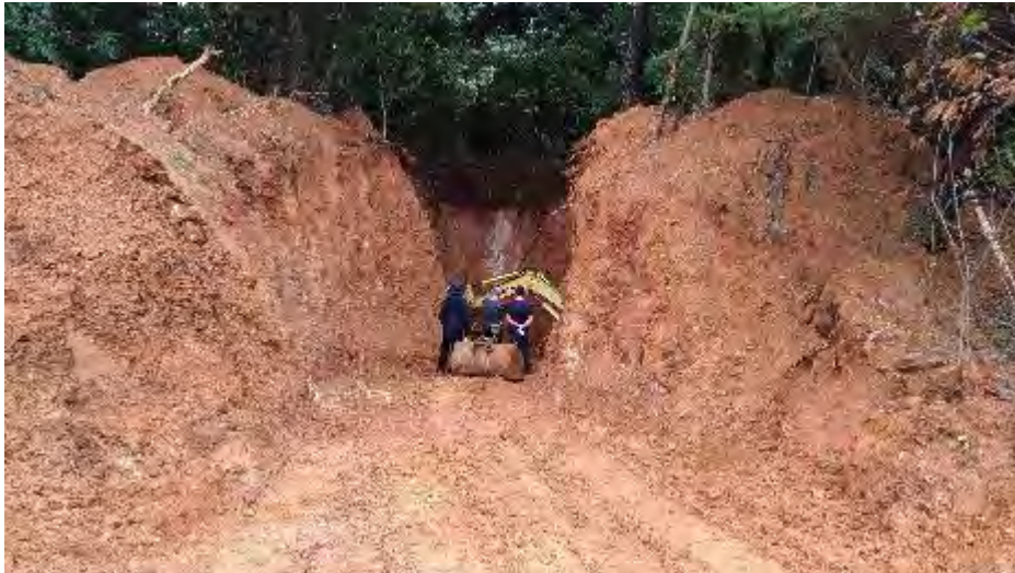
Figure 10.2: The Track to access the Main Inclined Shaft below the Concrete Collar at Gubong.
