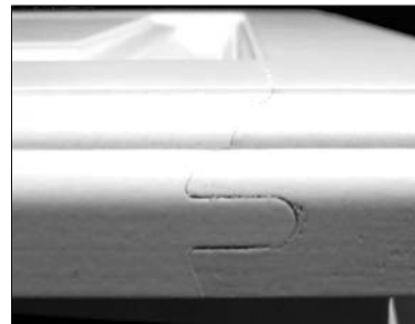
Example of end joint separation
