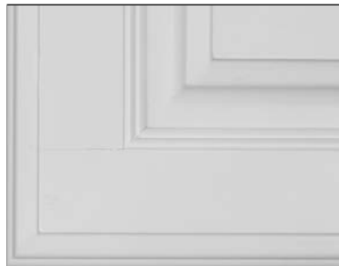
Example of front joint separation
