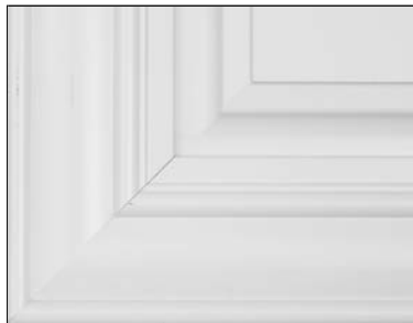
Example of front joint separation
