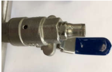
Downstream pressure vents in closed position
