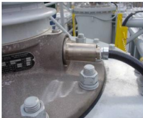
Fig.5. Installed Bushing Sensor
