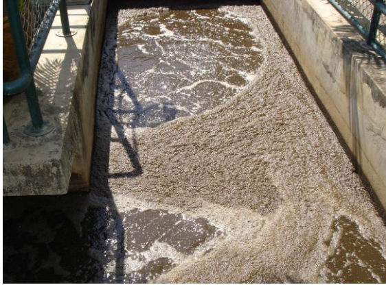
Fig.1. Aeration tank of wastewater treatment plant
