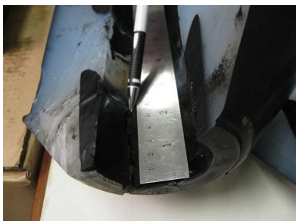
Figure 6. Damaged cable joint (B-phase)
