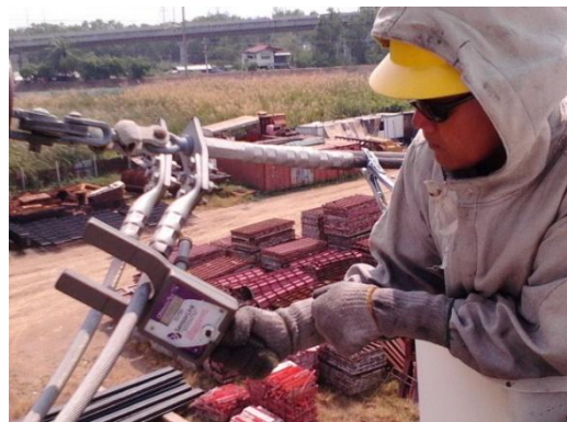
Fig.2. Contact measuring with live line micro ohmmeter
