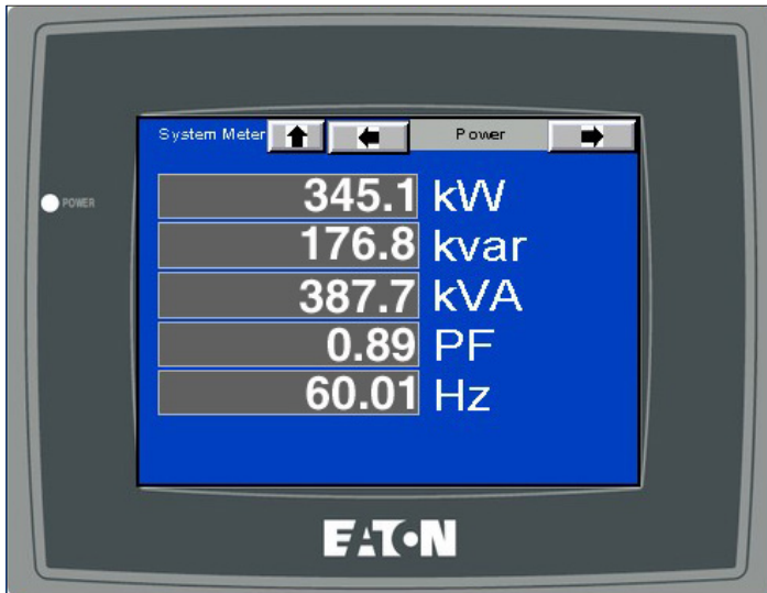
Figure 78. The System Meter - Power Screen.
