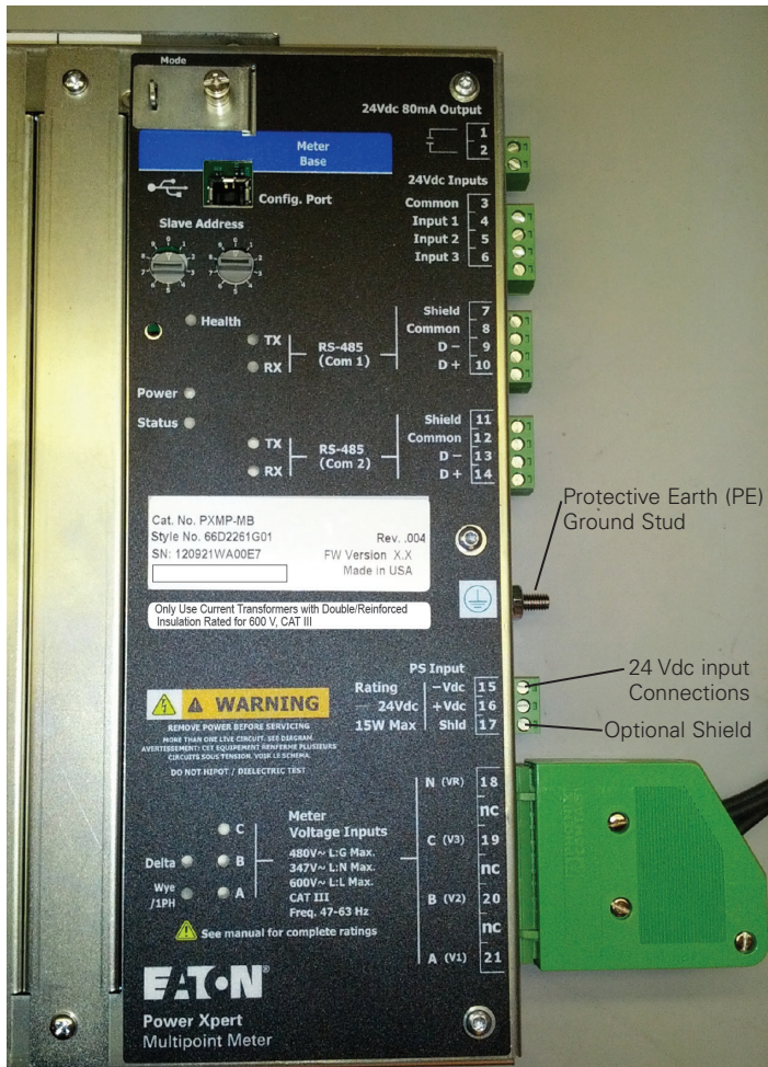
Figure 6. 24 Vdc Input, Shield, and Ground Connections on the Meter Base Assembly.
