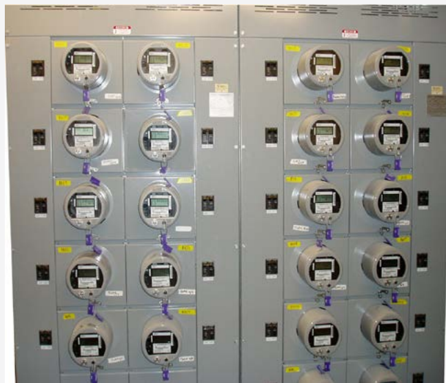
Service Disconnect, House Disconnects and Individual Apartment Metering
