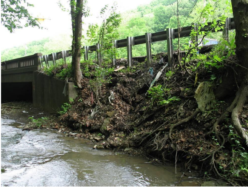
PHOTO NO. 7: Eroded Stream Bank/Roadway Embankment Just Upstream of Hutchinson Hill Bridge
