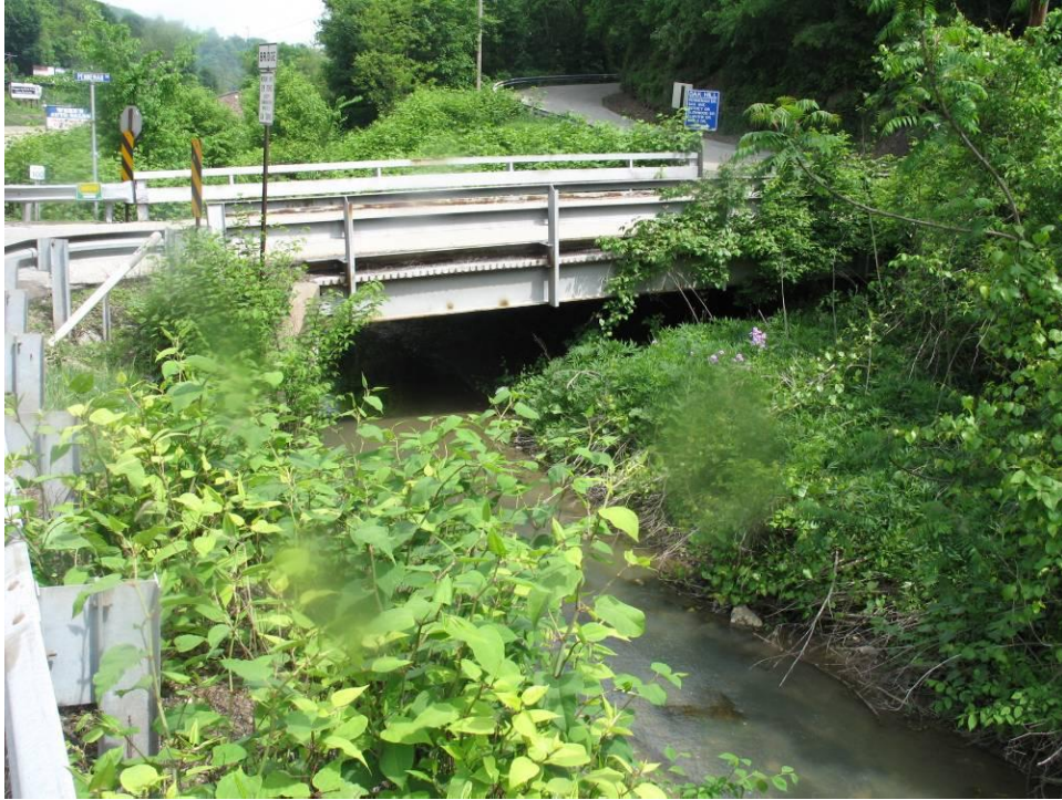
PHOTO NO. 21: Bridge Structure Downstream of Hutchinson Hill Bridge at Penneman Drive – Upstream Face
