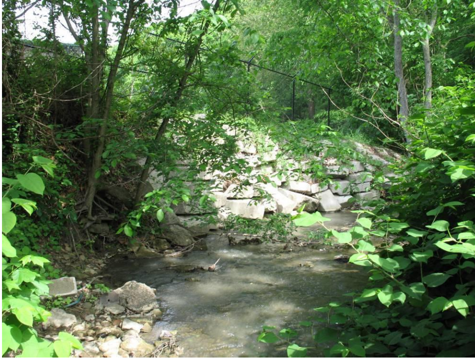
PHOTO NO. 19: Concrete Block Wall at Left Bank Approximately 350 ft. Downstream of Hutchinson Hill Bridge
