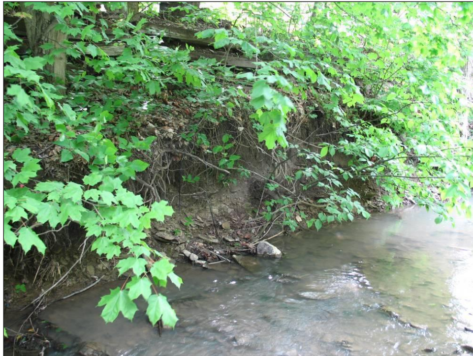
PHOTO NO. 26: Right Bank Scour Approximately 100 ft. Downstream of Hutchinson Hill Bridge; Timber Crib Wall Above.
