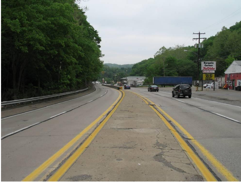
PHOTO NO. 1: South Approach Roadway (S.R. 51) to Hutchinson Hill Bridge (Facing North)
