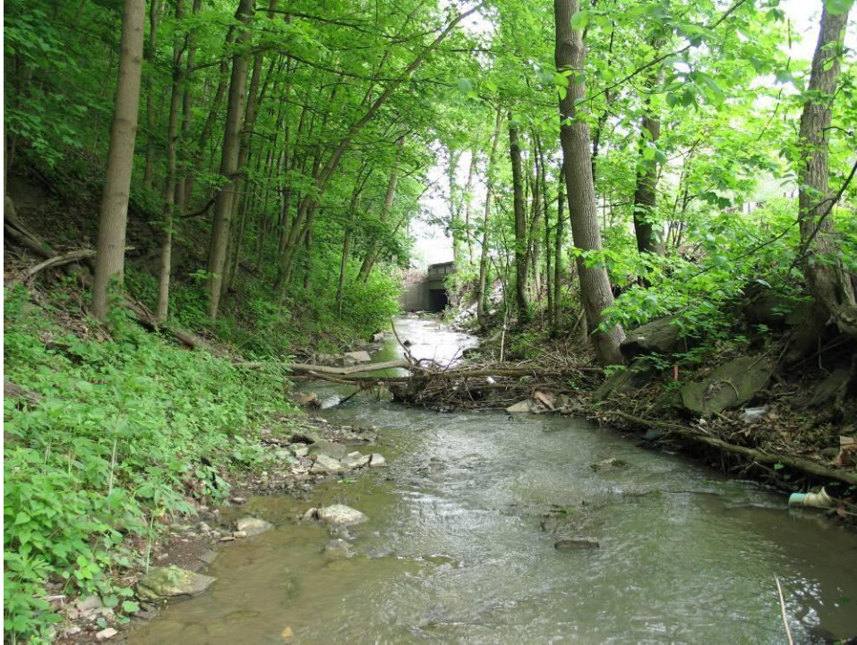
PHOTO NO. 9: Channel Approximately 300 ft. Upstream of Hutchinson Hill Bridge – Looking Downstream (Note Flood Debris in Channel)
