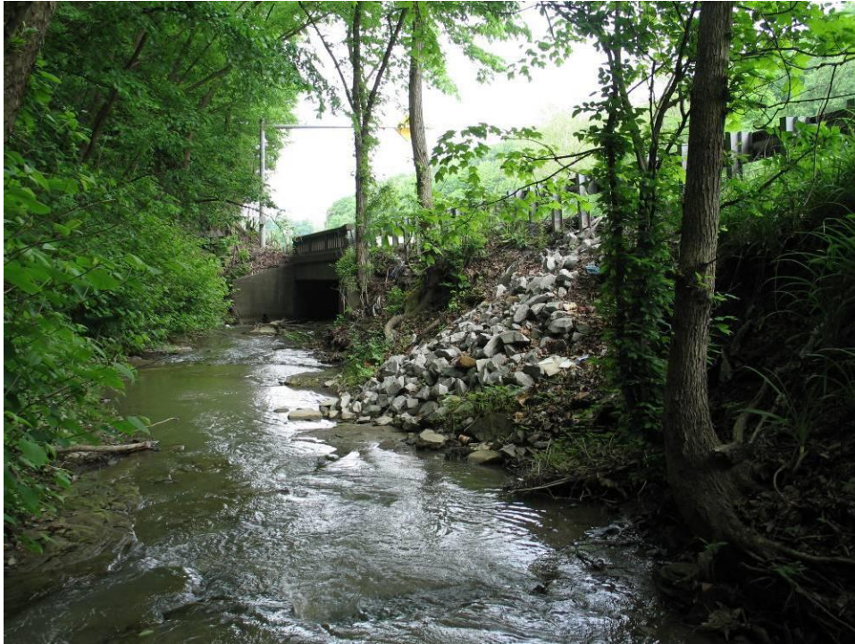
PHOTO NO. 8: Channel Approx. 150 ft. Upstream of Hutchinson Hill Bridge – Note Rock Protection on Stream Bank/Roadway Embankment.
