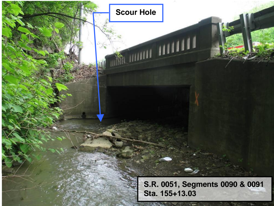
PHOTO NO. 3: Upstream Elevation of Existing Hutchinson Hill Bridge at S.R. 51 Over Fallen Timber Run
