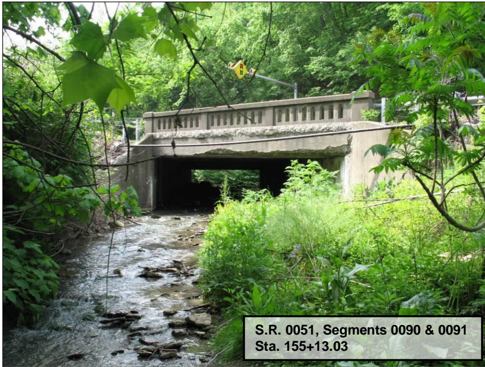
PHOTO NO. 5: Downstream Elevation of Existing Hutchinson Hill Bridge at S.R. 51 Over Fallen Timber Run
