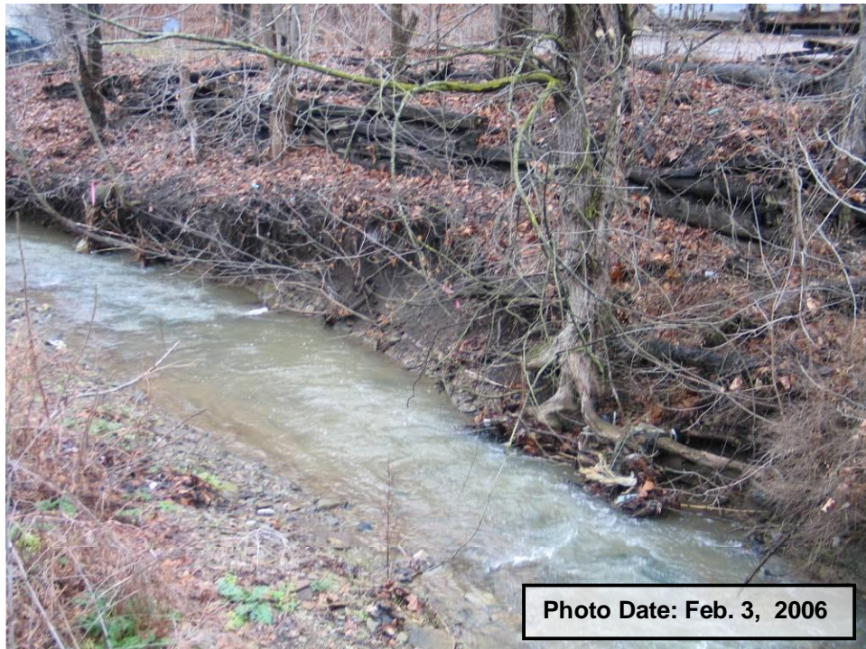
PHOTO NO. 30: Channel with Bank Scour and Timber Crib Wall Above it at Two Story Frame House Location (Photo 29).
