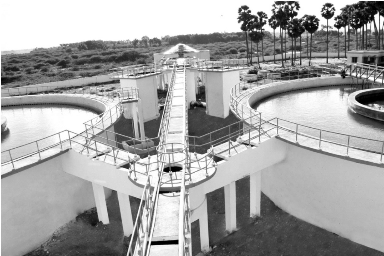
Water Supply Scheme to 755 Rural Habitations for M/s TWAD at Sattur, Tamil Nadu
