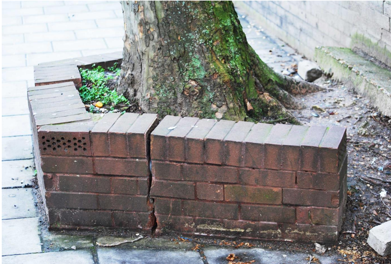
Image 4 – Many of the London Planes on Thurlow Street will require careful removal of existing hard surfacing and an assessment of structural root morphology where they have been in direct contact with built structures to confirm on-going stability
