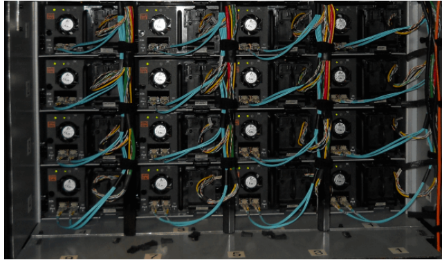
Figure 1-29 TS4500 drive bay
