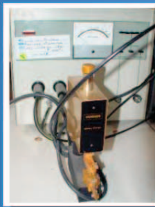
HUGHES WELD POWER SUPPLY & HED;MODEL #HRW-250; VTA 60 HEAD - ON PLATFORM
