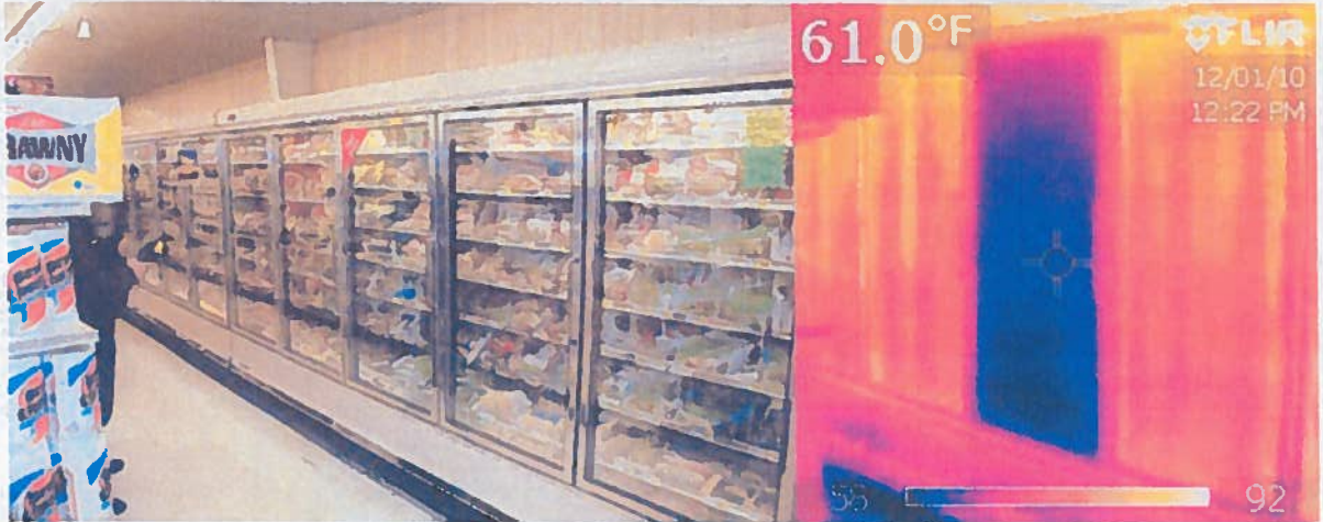
One of the case doors has lost the seal between the double pane glass, letting heat transfer into the refrigerated interior.
