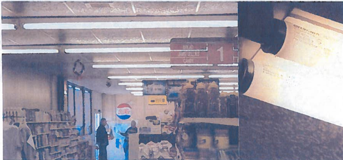
The store lighting is the older T12 technology. As ballasts fail these should be converted to T8 lamps with electronic ballasts.
