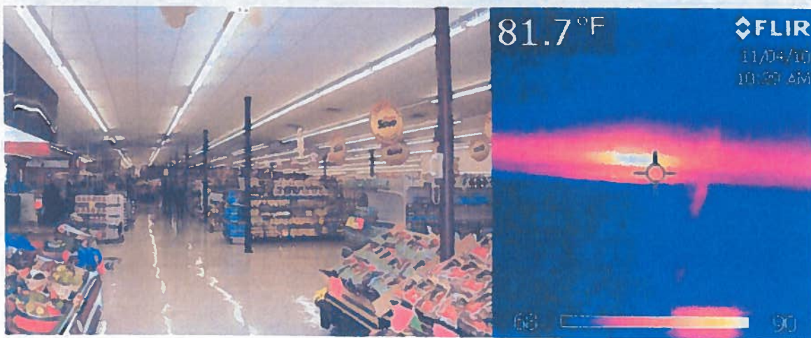
The fixtures are old style T12 lamps with magnetic ballasts.
