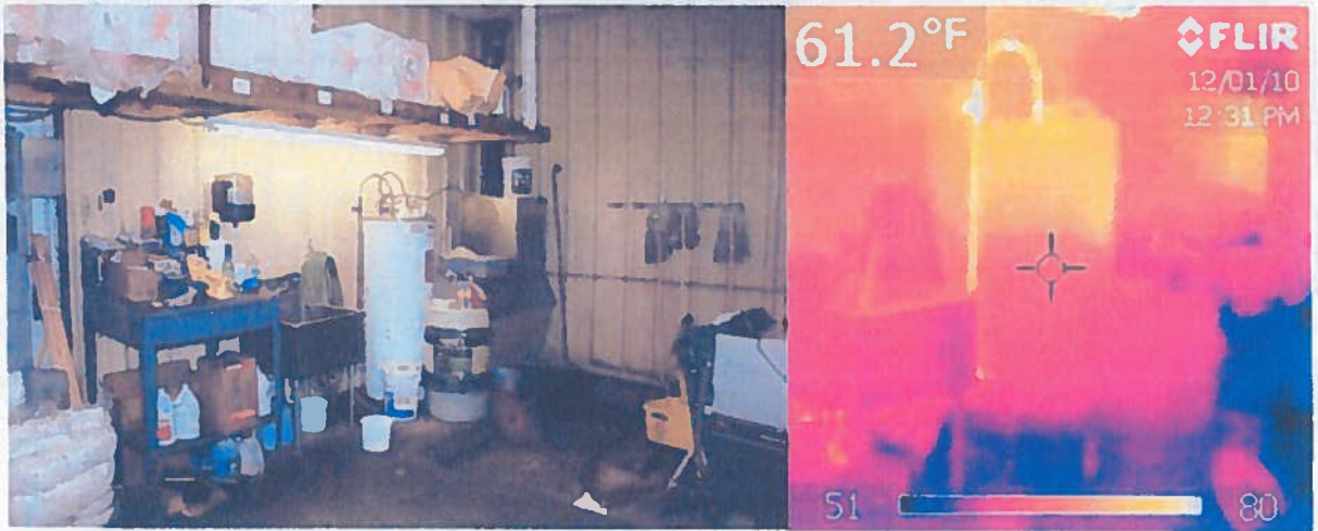
The electric water heater appears to have a bad lower element so that hot water only resides near the top.
