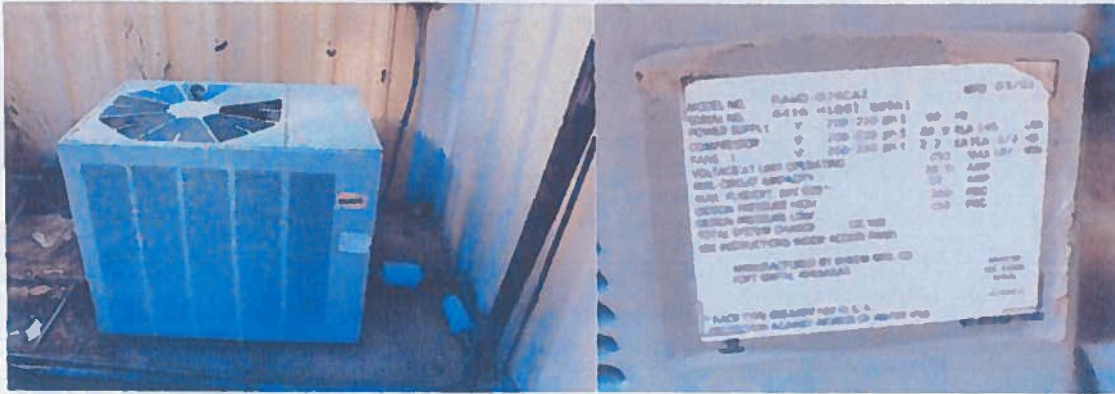
This split system air-conditioner dates from 2001 so is about 75% through its expected life.
