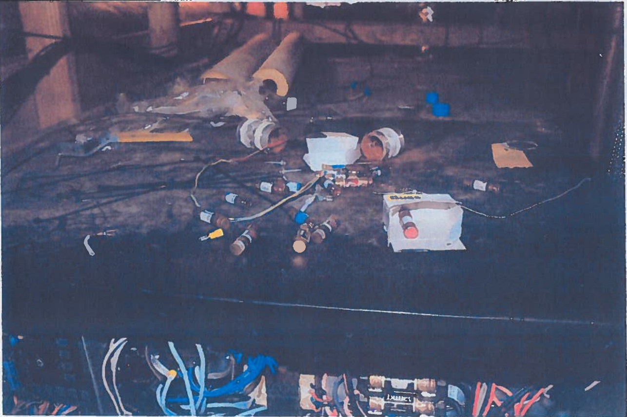
There was evidence of compressor overloads, requiring multiple fuses to be replaced.
