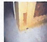
Incorrect Energy Corner
