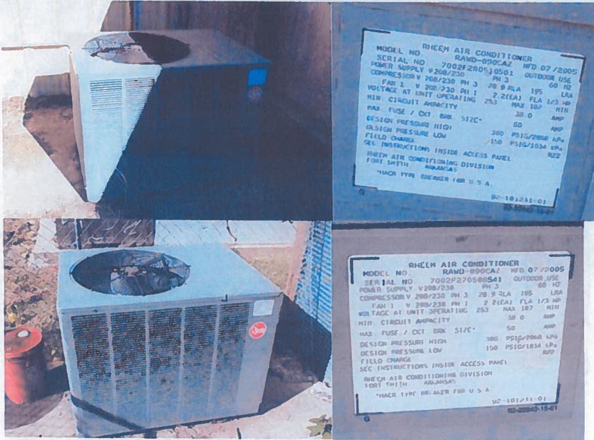
These split system condensing units are newer and date from 2005.
