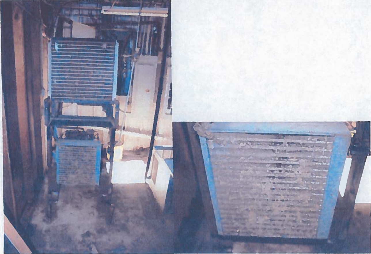
Examined the refrigeration equipment, noting that some of the coils were dirty and needed cleaning.
