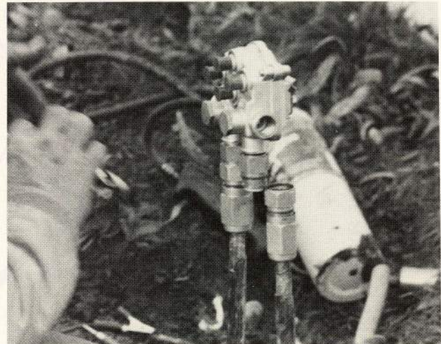
FIGURE 9/ installation of TX 'high frequency' multi-tap device on 0.500" cable 'risers' in buried cable plant.
