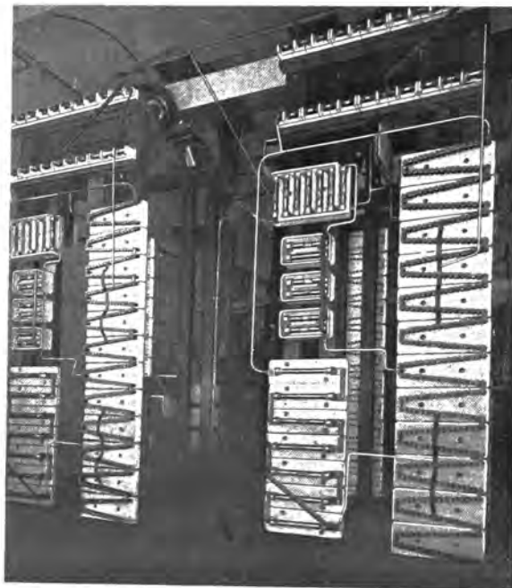
LIGHTNING ARRESTER COMPARTMENT OF PORTABLE SUB-STATION SHOWN ON PAGE 1
