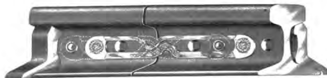
T Rail Double Bonded with Form A-8 Ribbon Bonds Spanning Both Inner Bolts
