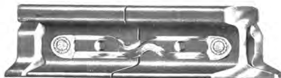
T Rail Bonded with Form A-7 Ribbon Bond Spanning Both Inner Bolts
