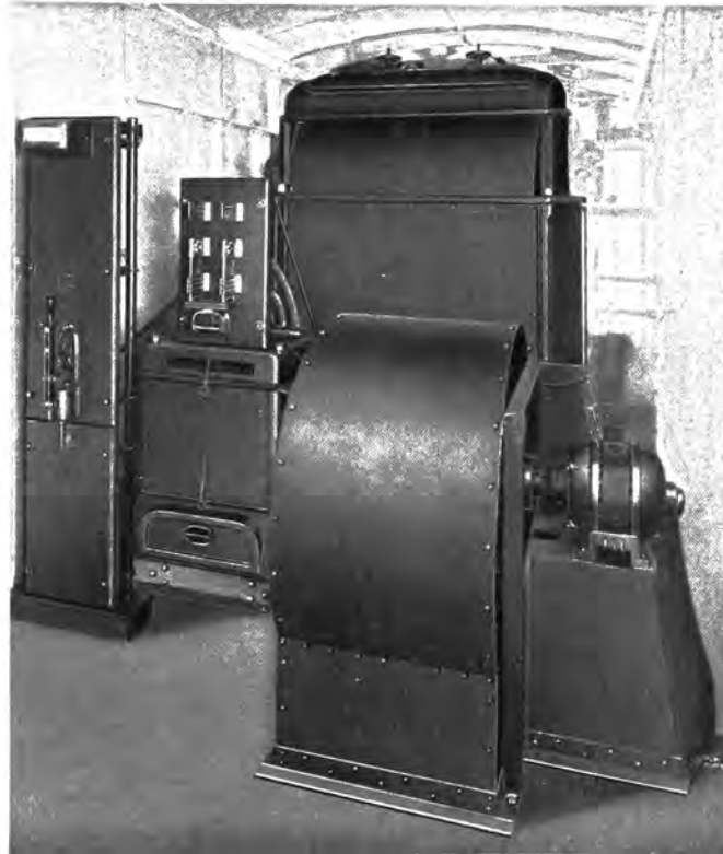
TRANSFORMER END OF PORTABLE SUB-STATION, 400 KW. CAPACITY, 33,000 VOLTS
