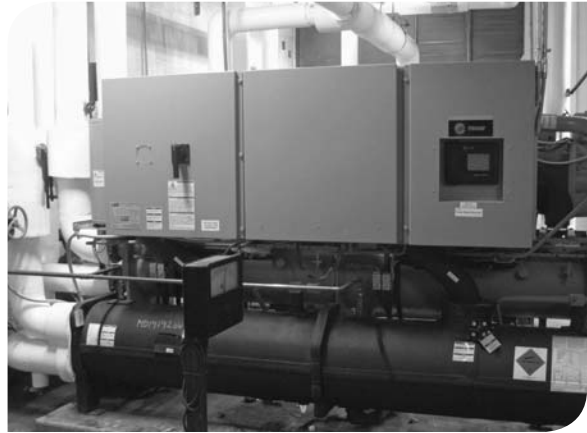
A new 100-ton high efficiency Trane water-cooled chiller saved Homestead-Wakefield Elementary 10 percent in electricity in its first summer of operation.
