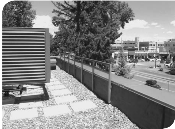
A Trane rooftop unit was installed on the second floor loading dock overhang to reduce installation costs and maintain building aesthetics.
