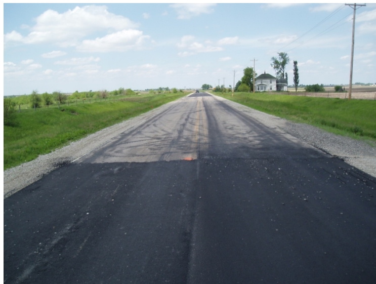
Figure 20. The gap in the HMA bond breaker where the geotextile material was placed
