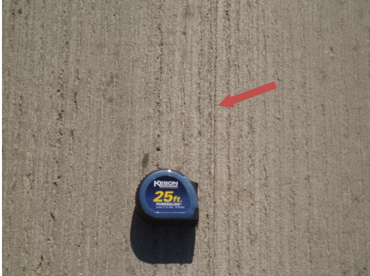
Pavement where a crack has formed along the longitudinal joint, but remains tight
