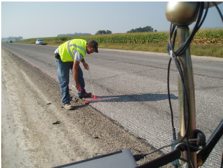
Figure 14. Worth County existing condition after milling
