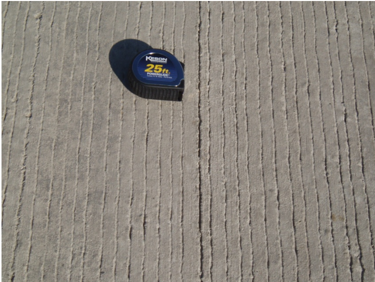
Pavement where a crack had formed along the longitudinal joint
