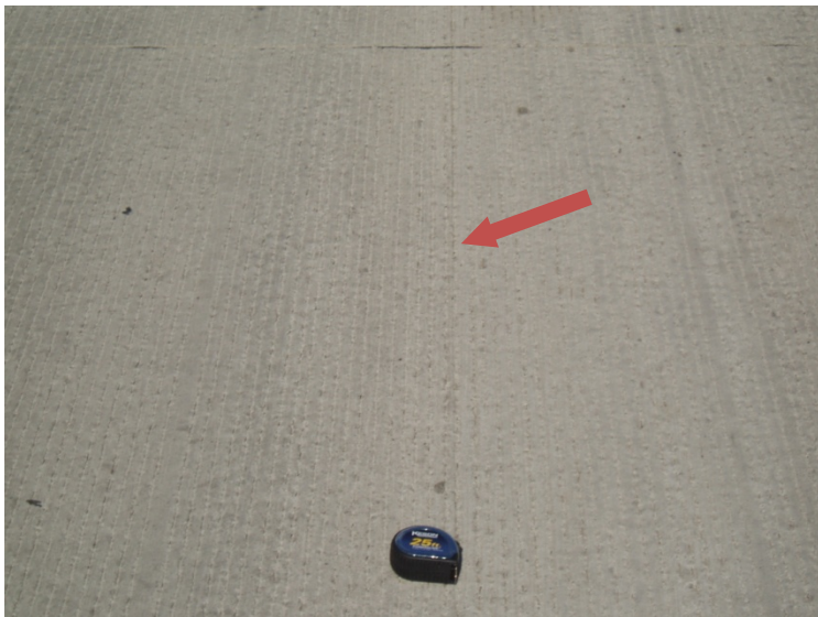
Pavement where a crack has formed along the longitudinal joint and is barely visible
