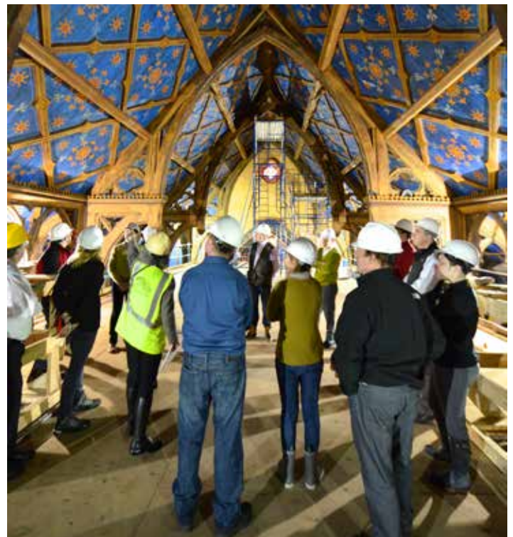
A hard hat tour of restoration work at Grace Church in Brooklyn Heights.
