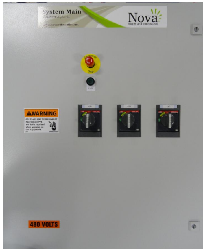
Figure 2 Nova NEA080AVWB Main Disconnect Panel- Outside
