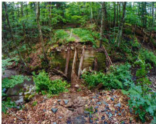
Collapsed bridge over the Charles Brown Bridge in 2018 (Photo by Doug Hardy)
