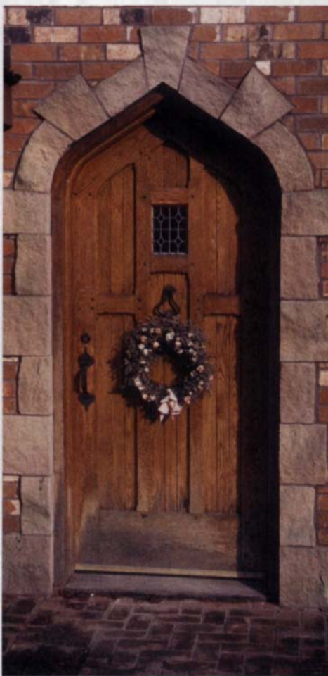
No finish lasts forever. This white oak door, built for a client seven years ago by the author and finished with six coats of spar varnish, shows the effects of exposure and neglect. The finish at the top of the door, protected by the overhanging wall, is still in good shape, but at the fully exposed bottom, the finish is completely gone.
