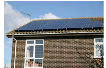
Figure 6.5. Solar photovoltaics: data from a 25\text{-m}^2 array in Cambridgeshire in 2006. The peak power delivered by this array is about 4 kW. The average, year-round, is 12 kWh per day. That's 20 W per square metre of panel.
