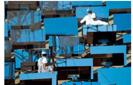
Figure 25.12. Two engineers assembling an eSolar concentrating power station using heliostats (mirrors that rotate and tip to follow the sun). esolar.com make medium-scale power stations: a 33 MW (peak) power unit on a 64 hectare site. That's 51 W/m 2 peak, so I'd guess that in a typical desert location they would deliver about one quarter of that: 13 W/m 2 .
