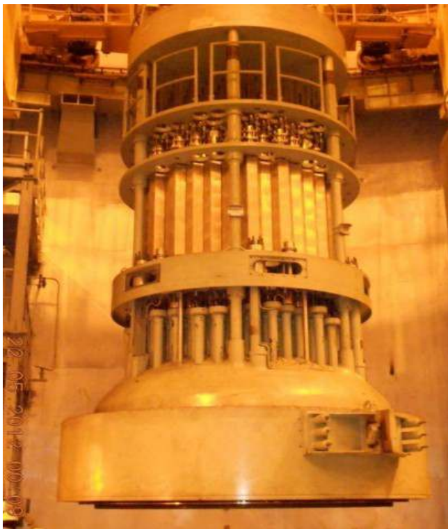
Top head of Reactor Pressure Vessel at KKNPP Unit-2
