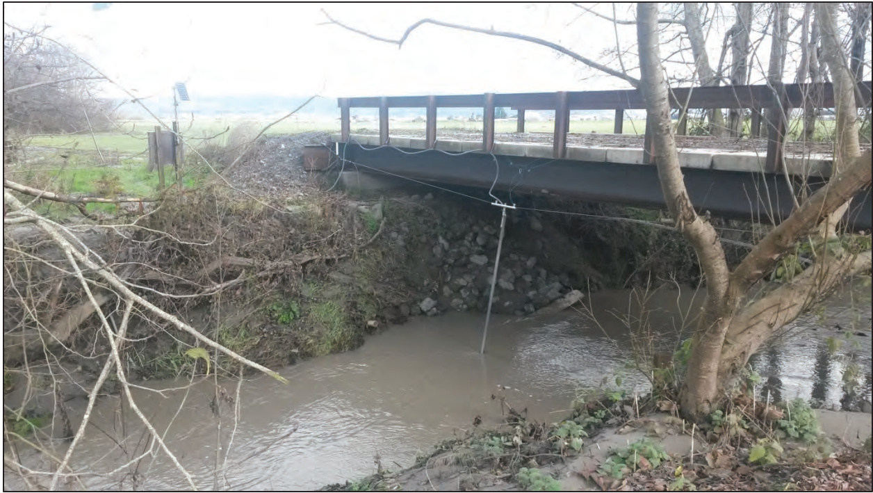
Figure 2. Upstream view of sampling section, turbidimeter boom on cable, gage house and solar panel.
