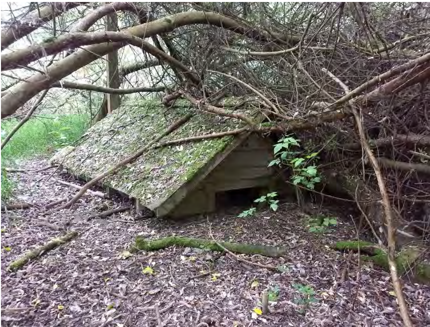
Figure 2-16. Buried outbuilding on south side of Williams Creek upstream of WCG-1 (Photo 2018).
