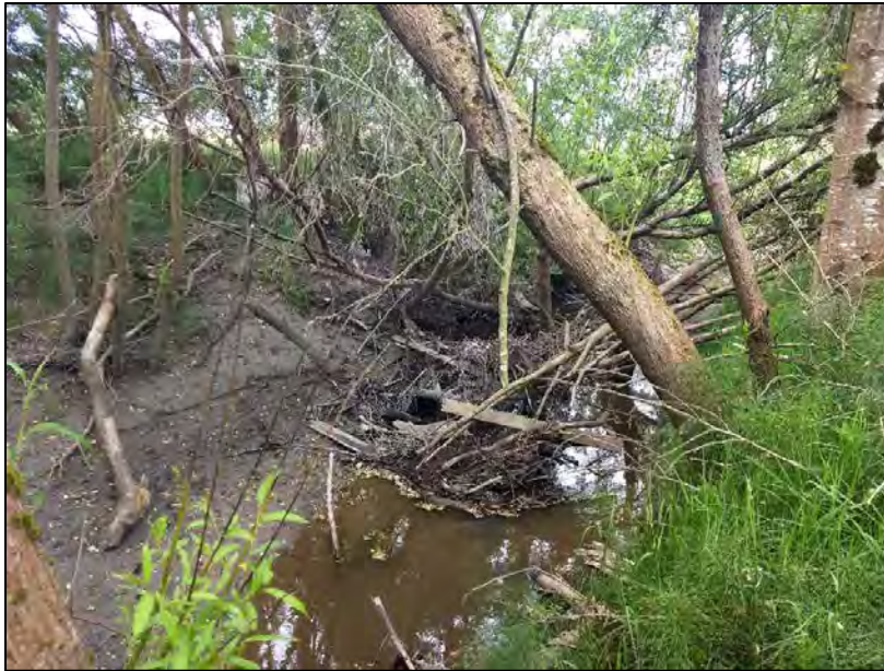
Figure 15. Overhanging trees and debris jam between Bridge 2 and Bridge 1 on Williams Creek causing sedimentation on the channel bed, banks, and overbanks.
