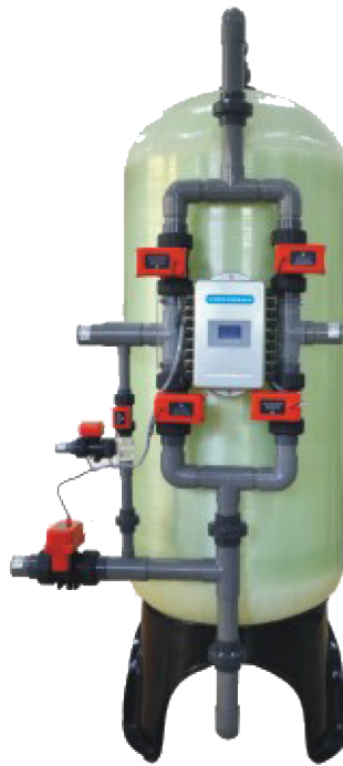
Softener control system
