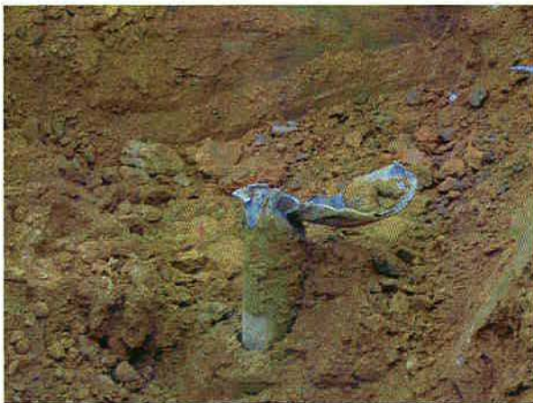
6-inch steel water supply well casing
