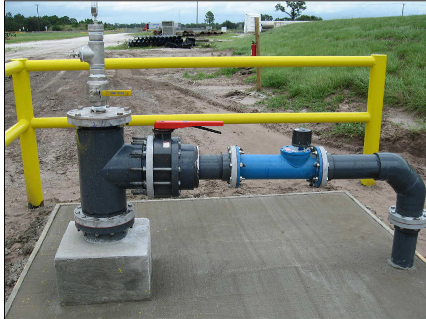
Figure 6. Wellhead and well pad.
