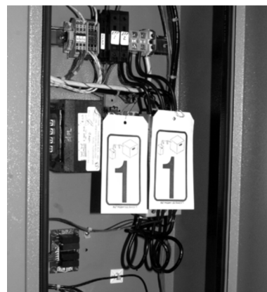
Figure 2: Reconnect Blower Contactor Coil Wires
