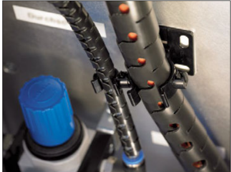
The protection and affixing of cables in a wiring cabinet with Helawrap sleeving.
