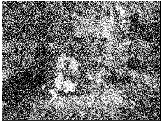
74. Pad mounted utility transformer outside south electrical room
