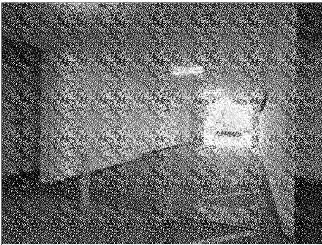
27. Surface mounted lighting at parking garage
