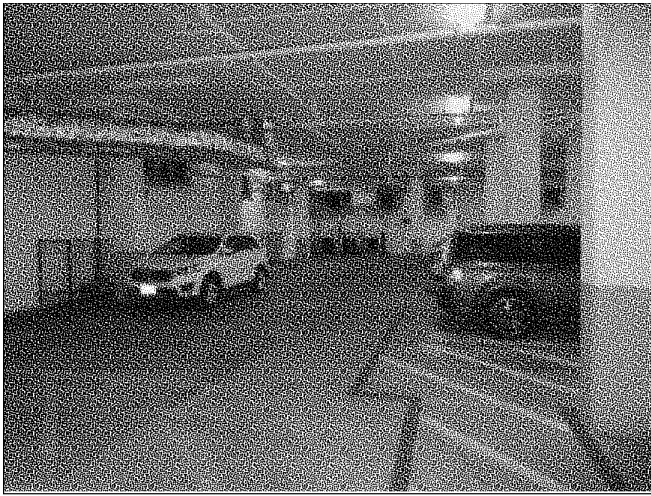
85. Fire sprinkler piping at the parking garage
