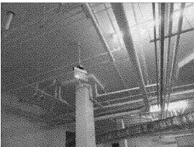
59. Drain and water supply piping for units above in the parking garage
