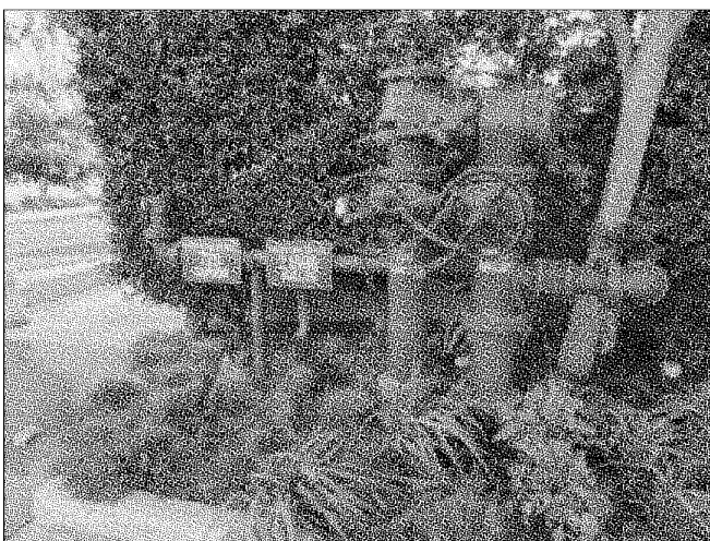
83. Fire supply with backflow preventor
