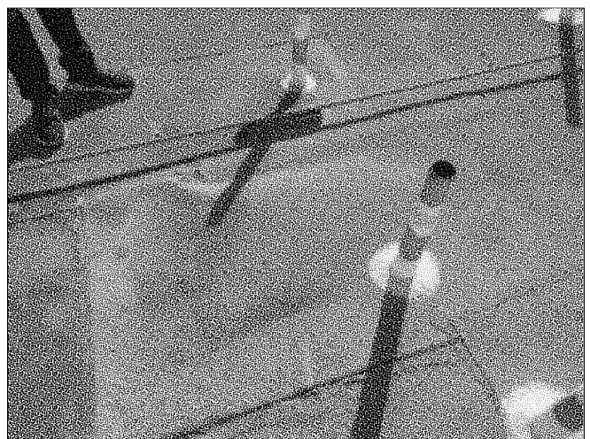
48. Blister at low-slope roof
