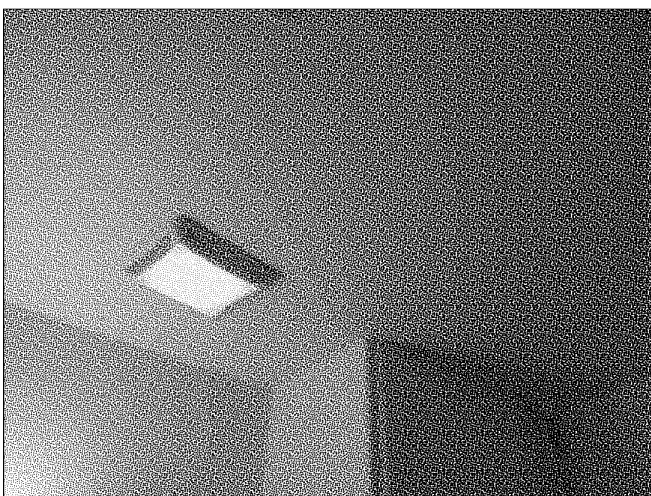
65. Exhaust fan at unit bathroom
