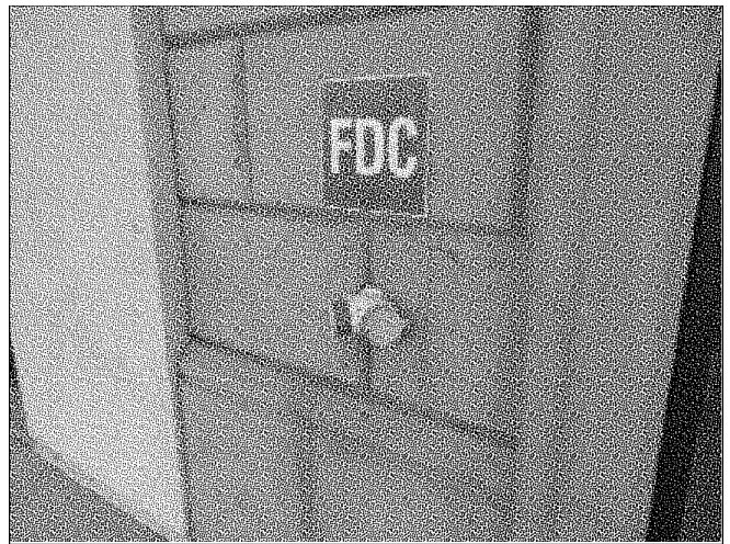
82. Fire department connection at main residential entry
