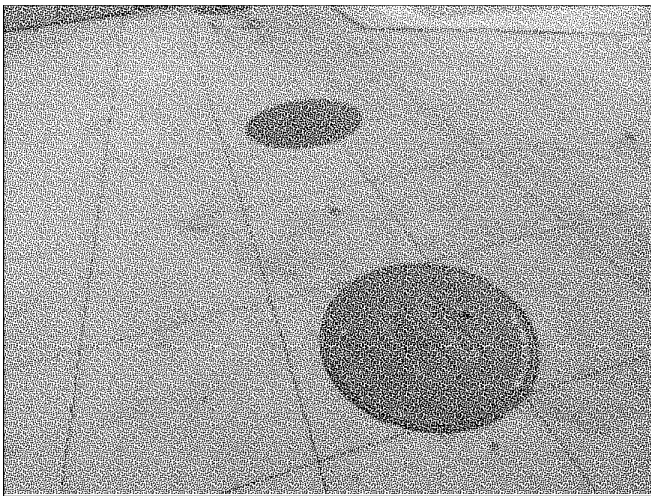
111. Holes in manhole cover exceed 1/2" diameter
