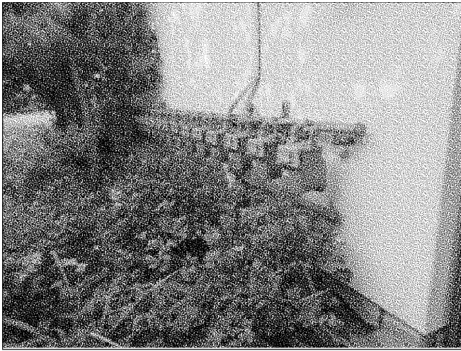
67. Gas meters for residential units
