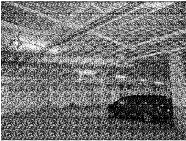
69. Kitchen exhaust duct in parking garage
