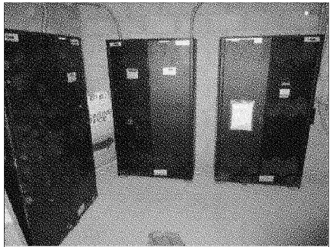
76. Battery inverters at electrical room
