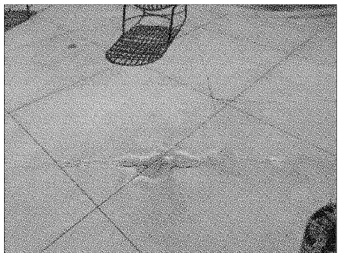
12. Damaged paving at swimming pool and spa
