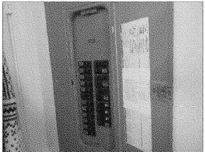
106. Electrical panel at unit
