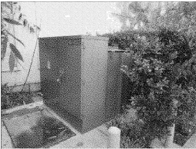
75. Pad mounted utility transformer outside north electrical room
