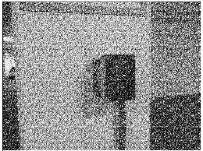
64. Carbon monoxide sensor for garage ventilation
