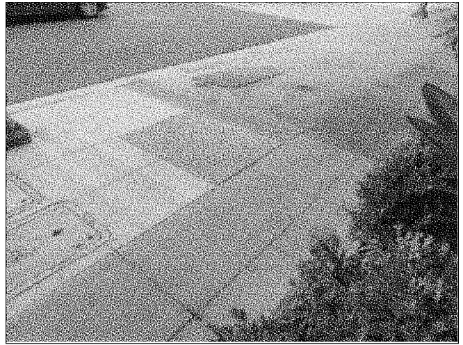
110. Detectable warning panels do not continue full width at the garage entry
