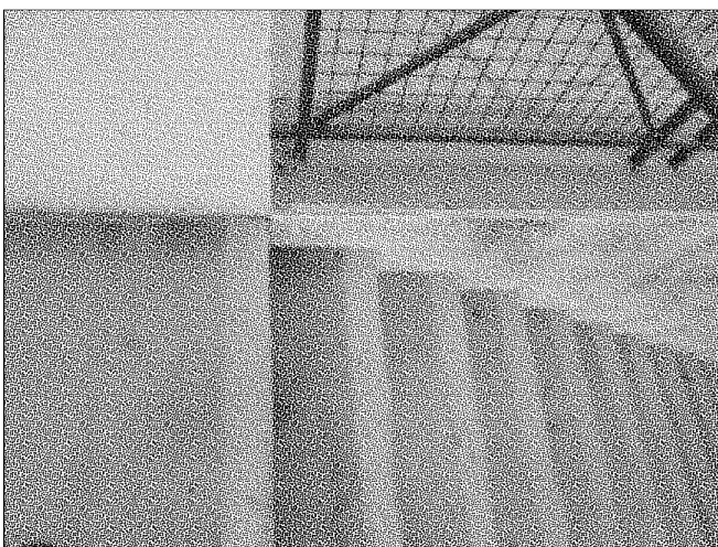
53. Steel framed concrete filled steel pan stairs from courtyard to street level
