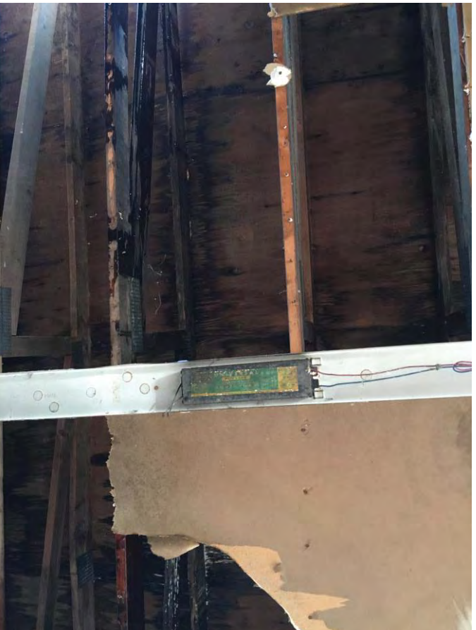
Photo 16: Suspect PCB-containing fluorescent light ballast in building 5/C (AOC-3/REC-3).
